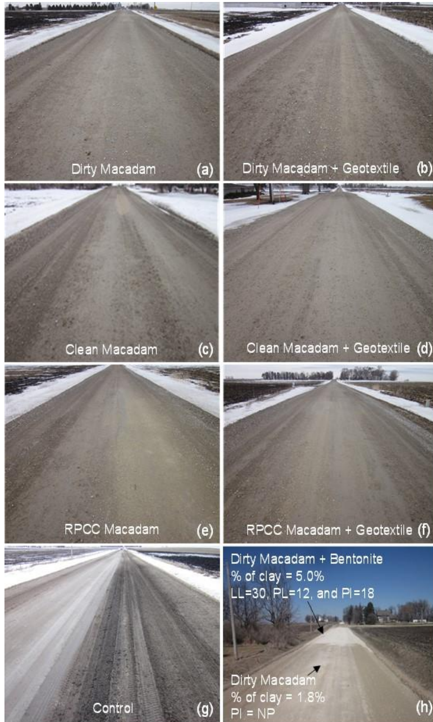
Figure 4.7. Surface conditions of (a through g) the MSB and control sections during the first thawing period (photos taken March 11, 2014), and (h) dirty macadam sections with and without the bentonite surface treatment during the second thawing period (photo taken March 28, 2015).
